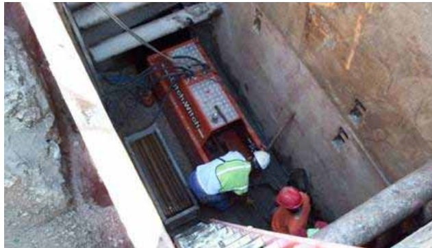
The Ditch Witch PR95 pipe bursting rig set up in a launch shaft.
