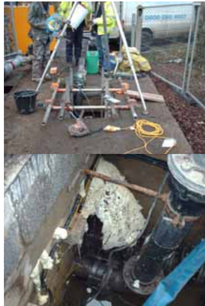
The shaft head set up for the wet well sealing project at Swallett Gate (top) with (bottom) gel used to seal the wet well at Swallett Gate shown having tracked back along the water channel into an adjacent valve chamber showing the route through which the wet well infiltration ran.
